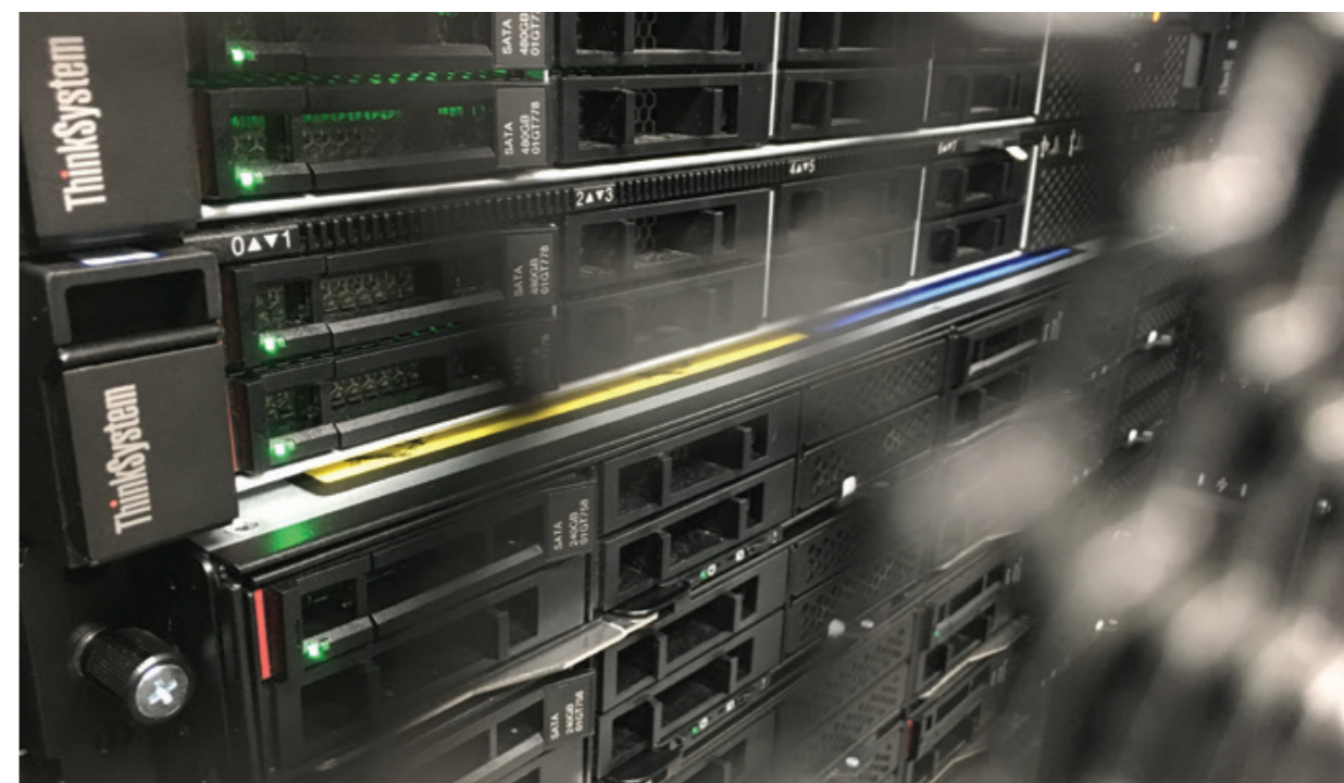
The new Hamilton cluster provided by Lenovo for data acquisition and data processing.
