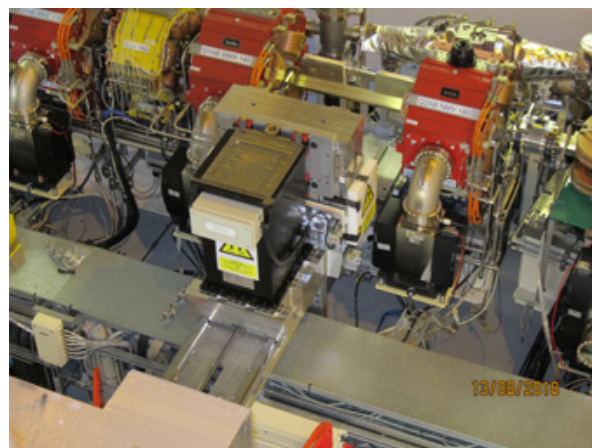
Figure 2: The girder with the 10-pole wiggler (the black object in the centre of the picture) in place of the “missing sextupole” installed in the storage ring. The wiggler is shown in its withdrawn position and was later moved over the vacuum vessel which can be seen behind the wiggler.
