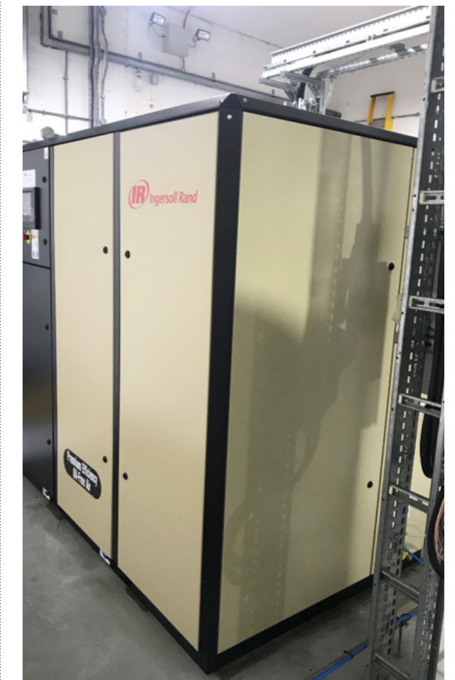
Figure 4: One of the two new variable speed drive air compressors.
